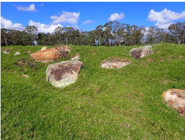
Figure 17 – Disturbed boulders on the side of the dam wall. View south.
